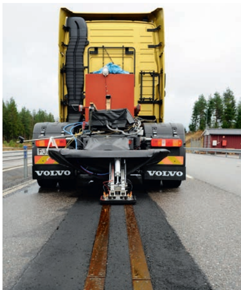
–Photos 3– APS ground power system on a Volvo test track in Sweden.
