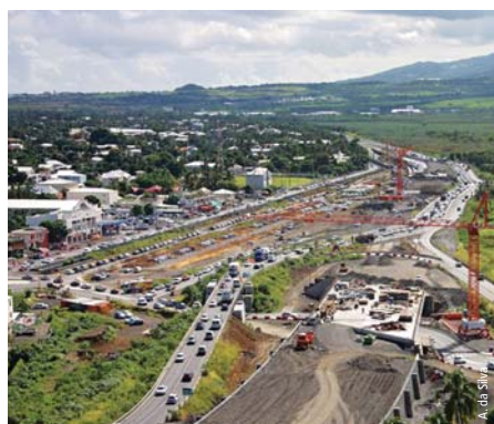
Diffuseur Saint-Paul centre, bas de Saint-Paul Saint-Paul centre, lower Saint-Paul junction
