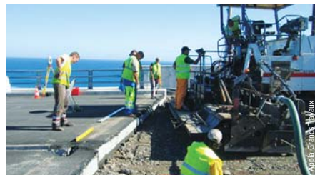
Photo 5 Redémarrage application graves non traitées réglage après ouvrage d'art Restarting, application of untreated roadbase aggregate and levelling after bridge structure
