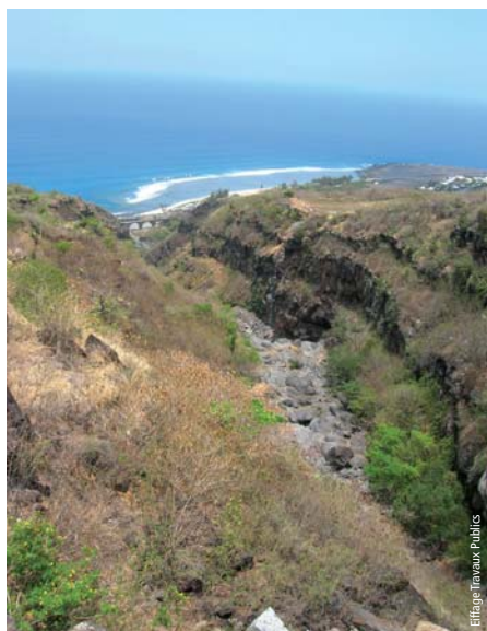
Photo 2 Ravine de l'ouvrage d'art non courant (OANC) 2 R 5 Ravine, non-current engineering works (OANC) 2 R 5
