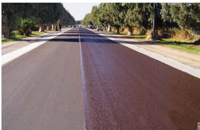
Photo 1 Application d'ECF sur la RN1 à Rabat Application of microsurfacing on highway RN1 in Rabat
