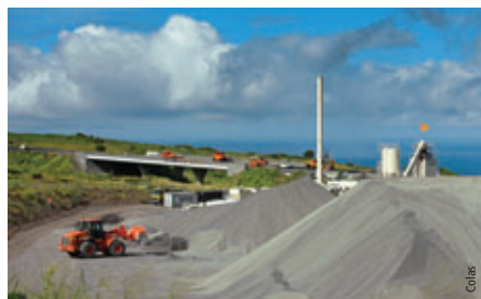
Photo 2 Centrale d'enrobage et stockage granulats Asphalt mixing plant and aggregate stocking
