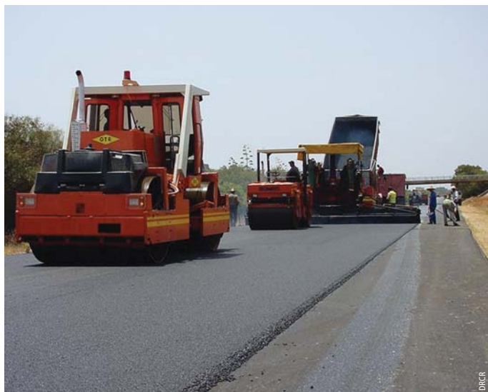
Photo 2 Application du BBTM en couche de roulement Application of very thin bituminous concrete on wearing course
