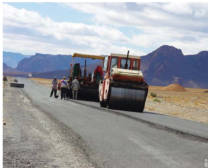
Photo 4 Application de la grave-émulsion sur la RN9 à Ouarzazate Application of emulsion-treated roadbase material on highway RN9 in Ouarzazate
