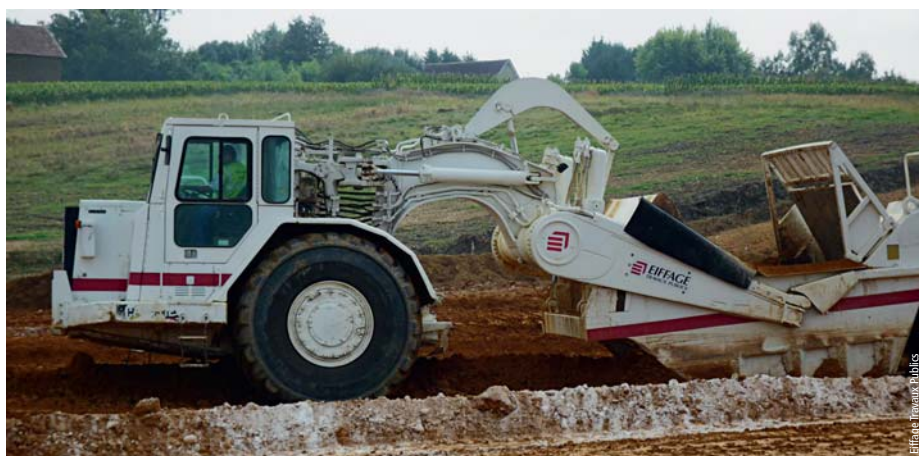
Photo 7 Moto-scrapeur sur le déblai D126 Motor scraper on cutting of highway D126
